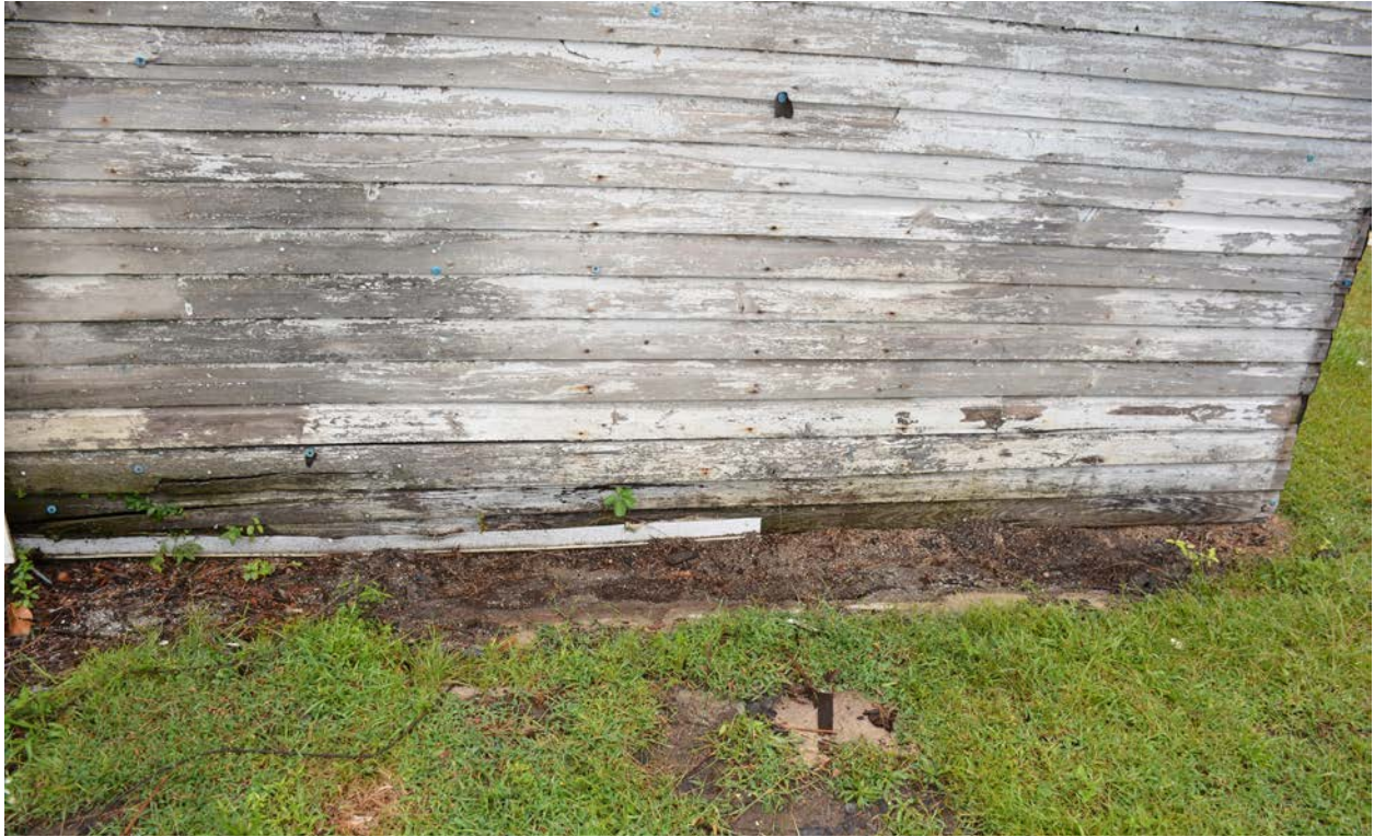
Water damage on the south section of the rear addition's west elevation (HF)
