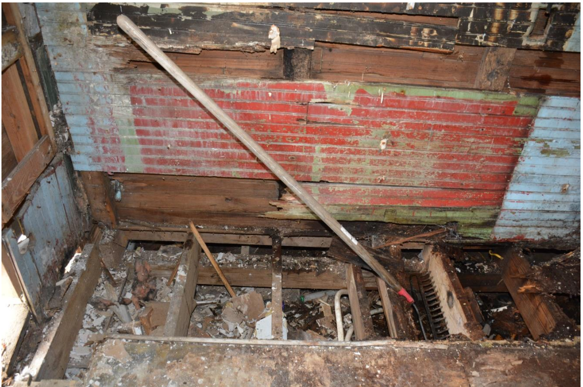
Kitchen floor damage under sink, August 2015 (HF)
