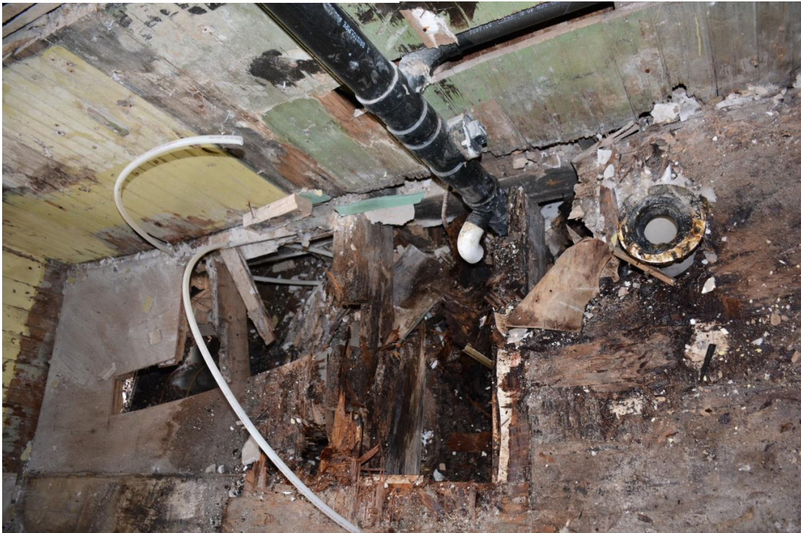
Bathroom floor damage, August 2015 (HF)
